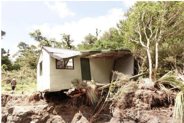
Leon Kinvig Hut destroyed by flooding of the Pohangina River due to Cyclone Gabrielle Pic from DOC
